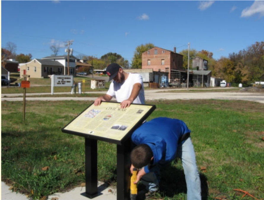
City of Union Maintenance Workers install Vitt's Mill Civil War Plaque at intersection of Highway 47 and Main Street.
