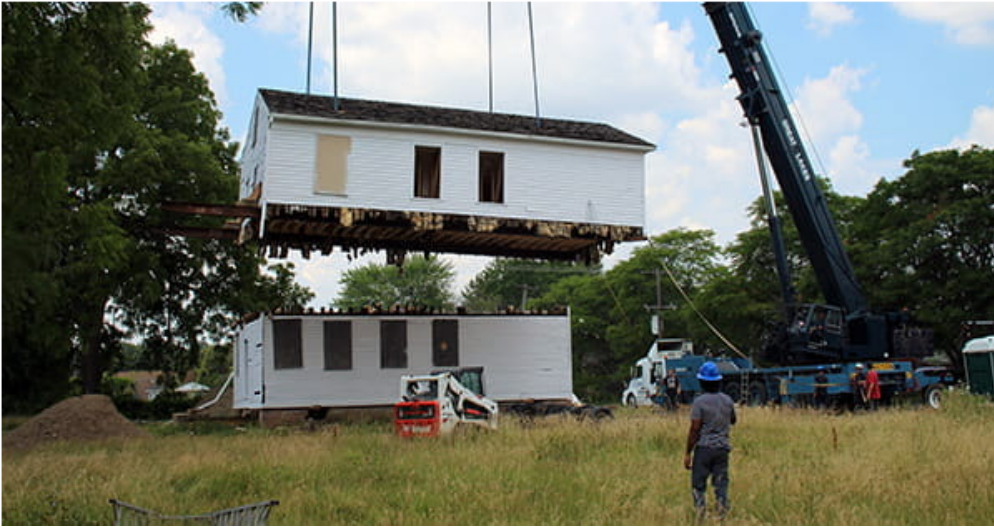
The first and second stories prior to loading on to two tractor trailers in July 2020.
