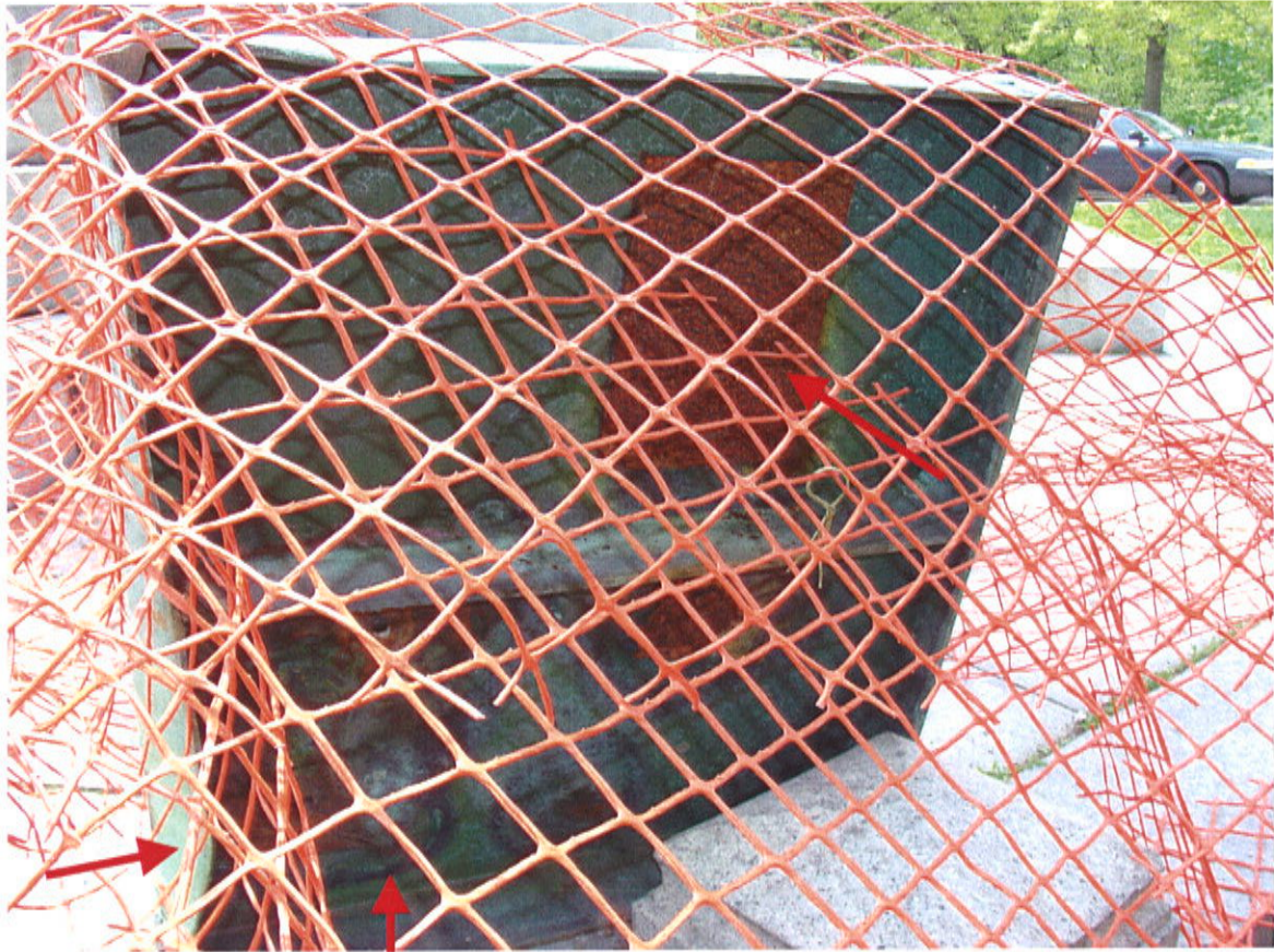
Shown: Soldiers and Sailors Monument, Boston, MA. Vandalized Soldier statue. Note: Base bent and damaged by vandals. Rusted plate is from a previous repair. Some corrosion and metallic stress damage.
