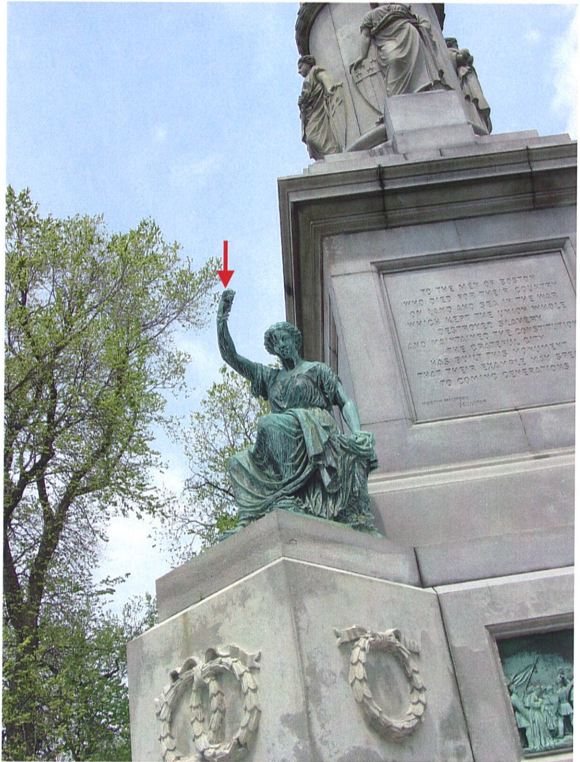
Shown: Soldiers and Sailors Monument, Boston, MA. Note: “Peace” statue missing part of olive branch, which extended from right hand. Some corrosion and staining damage.
