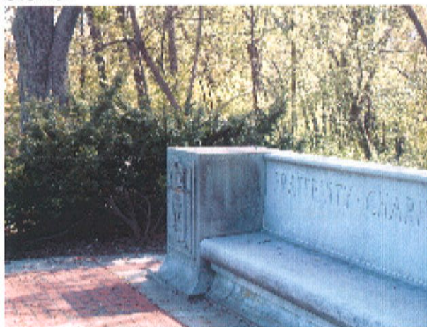
Fig. 11. Detail of the proper right side of the decorative wall/bench showing pins used for attachment of presently missing eagle.
