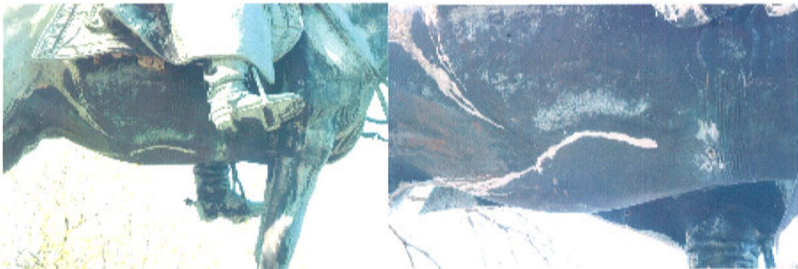
Fig. 4. Detail of the belly of the horse - showing streaking, mud wasp nests, and large areas of contrasting black, and green corrosion.
