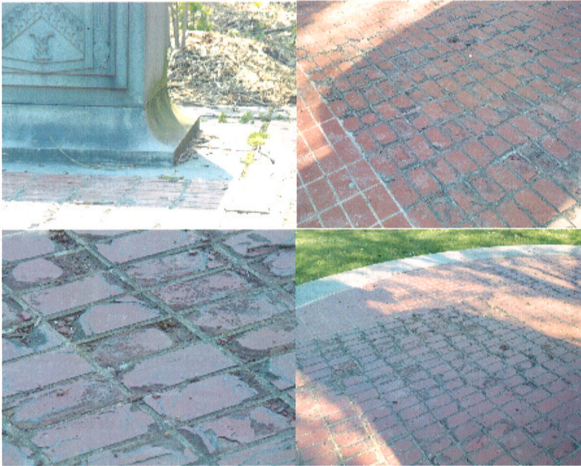
Fig. 15. Deteriorated pavement. These problems will not be included in the treatment proposal, because they can be dealt with by the owner. However, if requested we can address this problem also.
