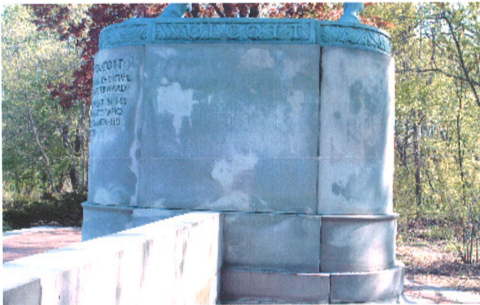
Fig. 9. Proper left side view of the pedestal with inscription. Please see discoloration of the stone. The staining is very uneven and disfiguring.
