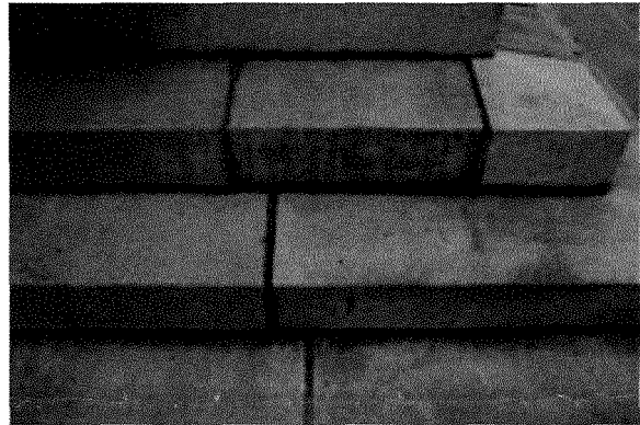
Steps show caulking issue.
