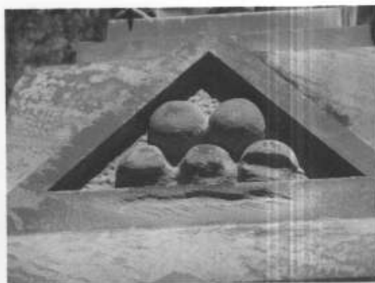
Damage to the cannon balls on the south face of the monument
