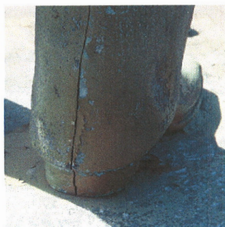
Crack in leg
