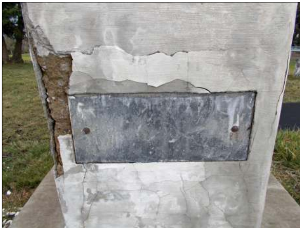
The concrete has split on the right side of the base. Inlaid tablets on both the right and left sides are missing.
