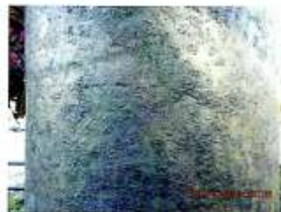
cannon shaft corrosion
