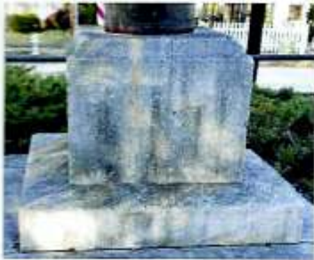
pedestal rust stains and mildew
